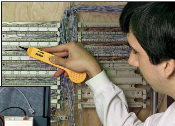
Trace phone/data wiring
